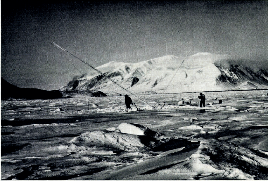
Fig. 4. Tower in process of erection. The use of the jib pole is clearly seen
