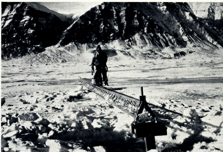
Fig. 3. Tower in horizontal position with wood platform for its base in foreground. The vertical projection is for attachment of a jib pole used to erect the tower. The mountains in the background are more than 5 km away
