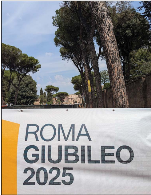
Figure 1. A screen conceals works underway on Via di S. Gregorio between the Palatine and Caelian hills, with the Arch of Constantine visible in the distance. Photograph by R. Witcher.
