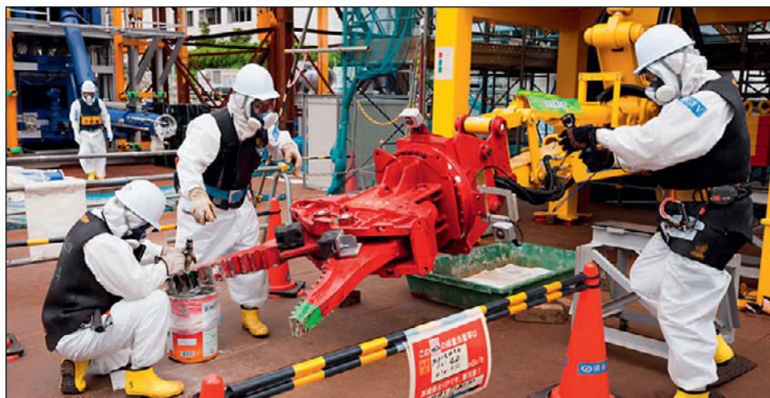
A device designed to grab up to seven tons of rubble to help clear debris from the Fukushima Daiichi site. It is in operation at Unit 1. Credit: Tokyo Electric Power Company Holdings, Inc.
