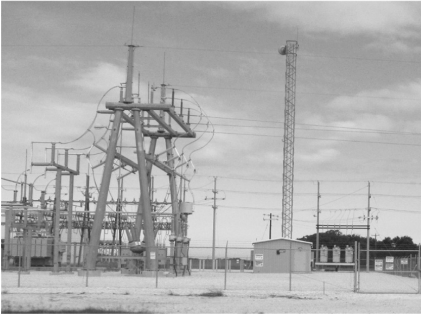
Figure 1.6 A communications microwave antenna belonging to the electric grid for transmitting sensing and control data on top of a tower behind an electric power substation control house on the right.
