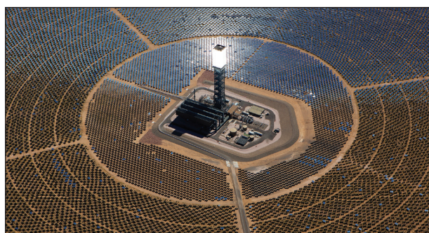
Mirror assemblies that focus the power of the sun on solar receivers atop power towers at the Ivanpah Solar Electric Generating System in California’s Mojave Desert. Credit: BrightSource Energy.
