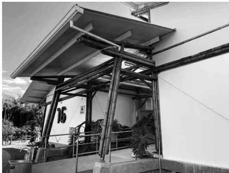
3 The bamboo species of Guadua angustifolia is well documented in the Colombia building code. Bamboo is the primary structural material in some campus buildings at the Universidad Tecnológica de Pereira, in Pereira, Colombia.
