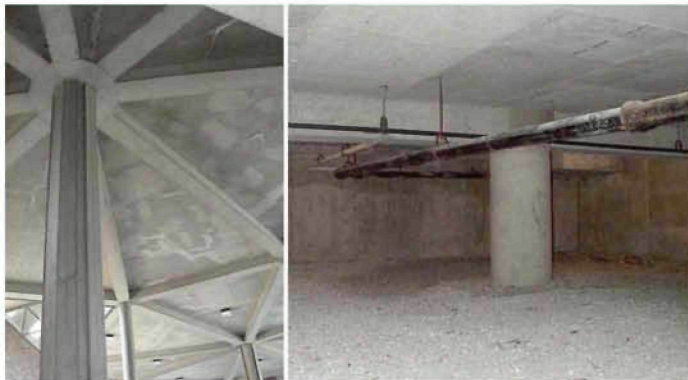
Figure 5. (Left) Radial beams supporting the floor above the STEM room and nearby labs. (Right) Space beneath the concrete floor slab that supports the JEOL JEM-2010F TEM/STEM. This picture shows the base of the building column, the asymmetric beam (running left-to-right across the top of the column) and the depressed 12-in thick floor slab of the exterior decorative wall indentation (appearing to the right of the column just behind the beam). The beam and 12-in thick depressed floor slab are indicated in Fig. 4 bottom as the dark purple line and gray-green square, respectively. The JEM-2010F is located roughly above the drain pipe where it passes behind the building column.
