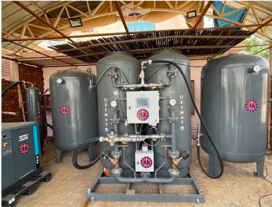
Figure 2. Pictures from the field. The PSA Oxygen plant installed.
