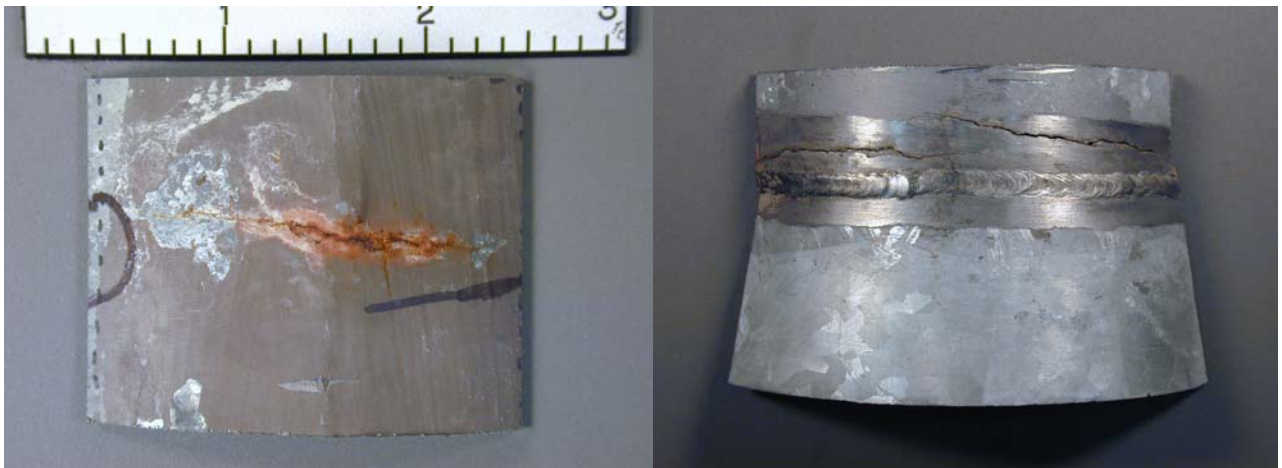
Fig. 1. Sections of pipe from vent system on waste tank. Cracks are in heat affected zones of welds.
