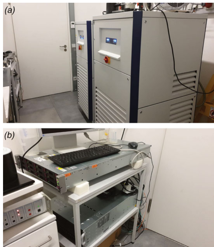
Fig. 6. Ancillary equipment room. (a) Water coolers for two TFS cryo-TEMs (Van der Heijden Labortechnik GmbH). (b) Servers for a Falcon 3 camera (top) and for a K3 camera (below).
