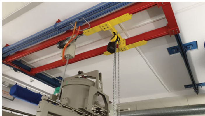
Fig. 10. Overhead crane for lifting heavy equipment. Crane with a 1000 kg capacity suitable for a 300 kV microscope. Such a crane is very useful for installation and servicing of high-end electron microscopes. However, most deliveries of large, high-end electron microscope now include a crane, sometimes even contained within the microscope housing.
