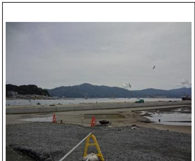
The main docks at the Port of Miyako, just beginning to be rebuilt, in September 2012.
