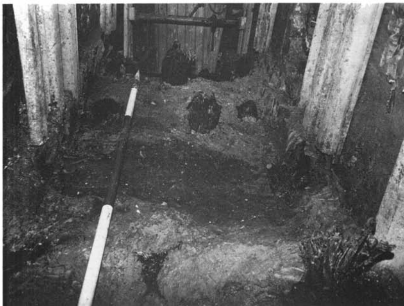
A. View of the upslope end of Trench 101 showing the undisturbed timber piles (the scale rod is divided into 50 cm lengths). (p. 216).
