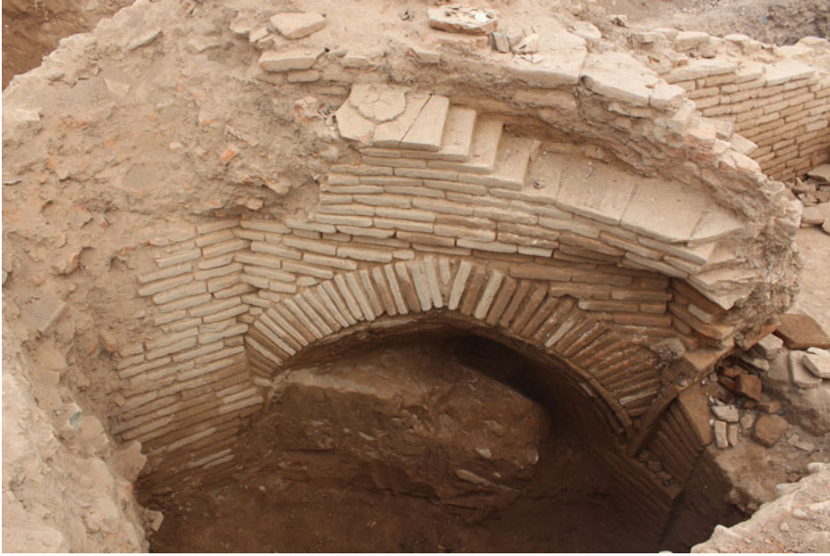
Figure 8. Remains of the foundation of the dome in the main burial chamber. Source: Photo by Kubatbek Tabaldiev and Kunbolot Akmatov.
