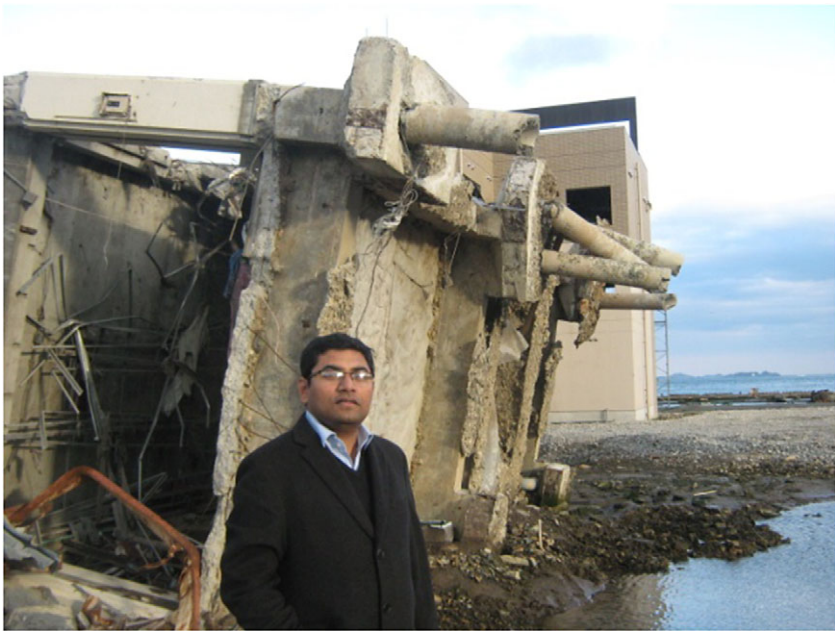
Figure 11. Collapse of the pile-supported building following the same 2011 Tohoku earthquake.
