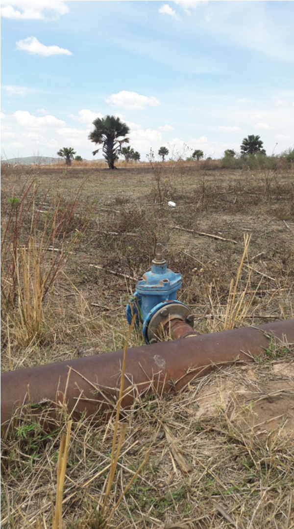
Figure 2. Rotating taps for sprinkler irrigation.
