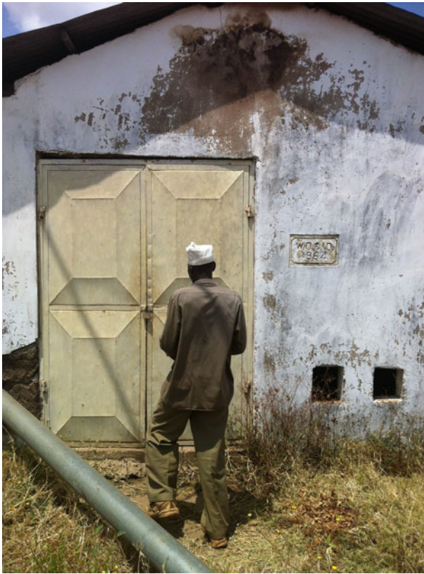
Figure 4. One of two pump stations, carrying the insignia ‘W.D. & L.D. 1964’.
