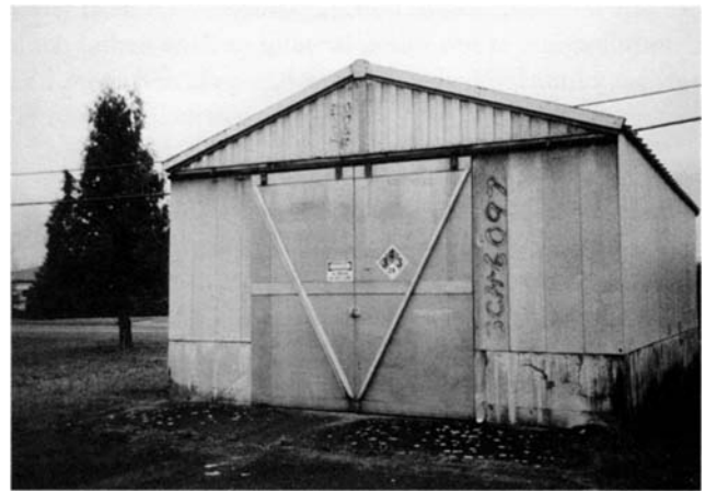
Figure 3. Oil Storage Building that previously contained unlabeled, leaking hazardous waste containers, North Pacific Division Laboratory, Troutdale, Oregon.
