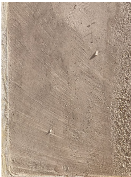
Figure 8. Polished opus signinum surface repelling water droplets. Note the trowel marks left in the process and the rougher, washed off surface, showing the difference between original finish and ‘archaeological’ state.
