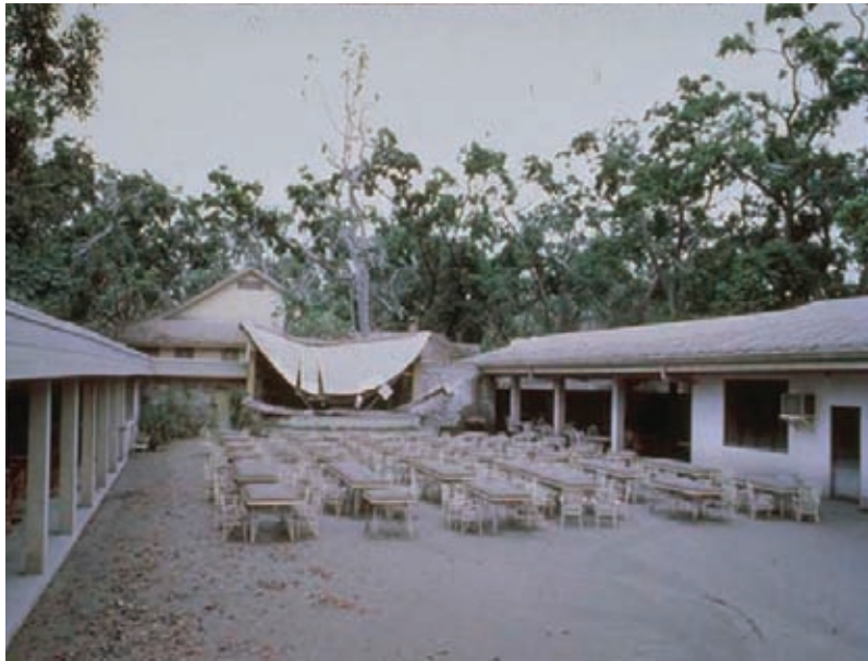
Collapse of a weak metal sheet roof under 150 - 300 mm of ash during the 1991 Pinatubo eruption, Philippines ©T.J. Casadevall, USGS.
