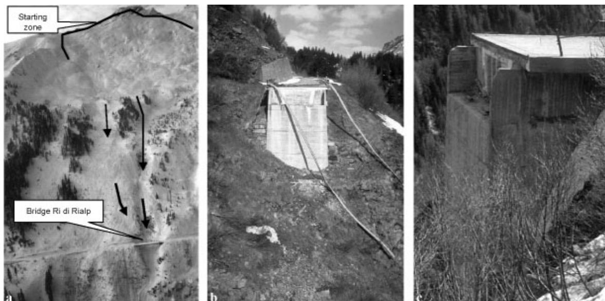
Fig. 3. (a) Overview of avalanche track and bridge Ri di Rialp, avalanche from January 1994. (b) Destroyed bridge with unfastened rail guards: view to abutment B, May 1998. (c) Abutment A with undamaged wing walls, May 1998.
