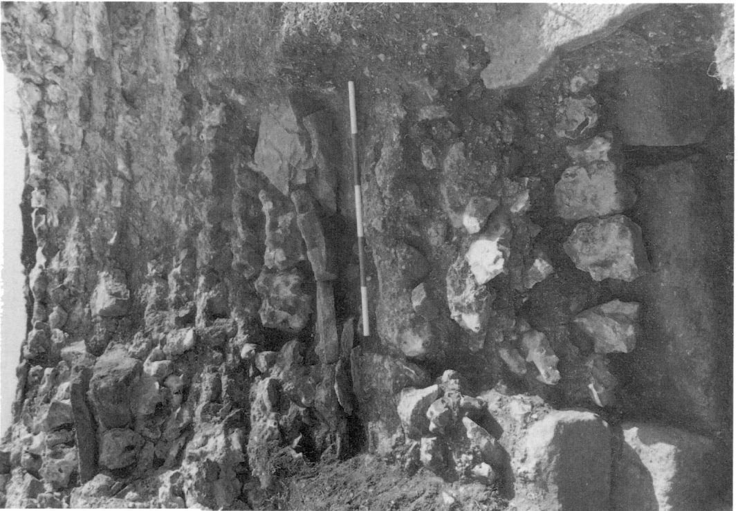
(Photo: M. Fulford) A. Silchester Town Wall 1992: Trench 1: remains of wall from the outside showing subsidence and possible gang junction. (p. 142)
