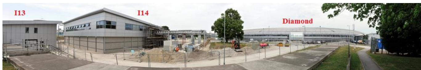
Figure 1. Panoramic view of the I14 and electron microscopy building under construction at Diamond.
