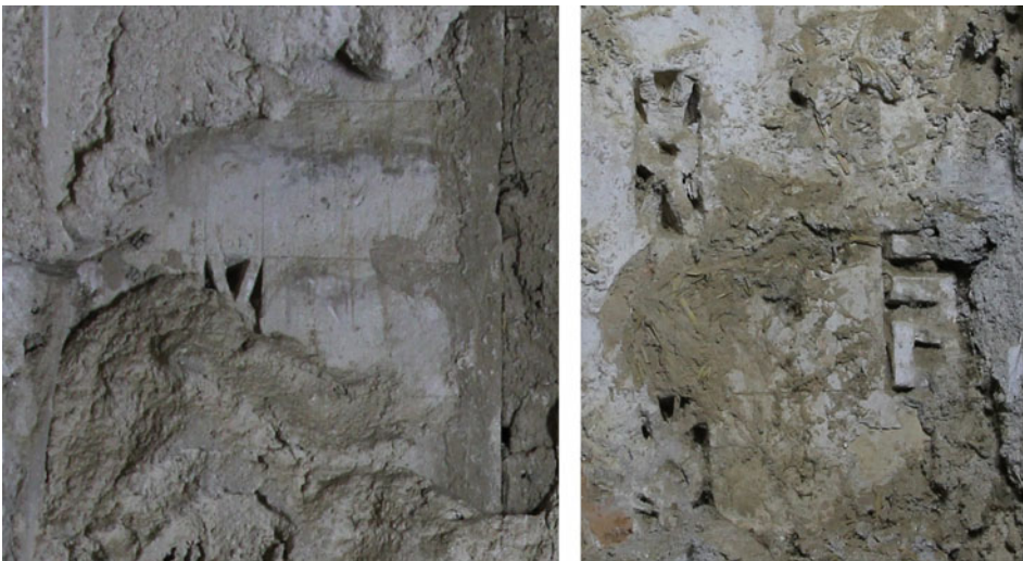
Fig. 8. Incised construction lines in the earliest phase of brick decoration to the right of the mihrab niche (L), and square Kufic Allah brick plug (R).
