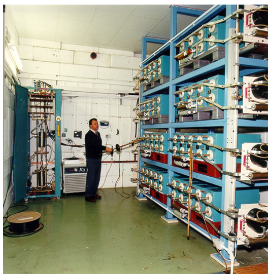
Figure 66. The CLF's Ray Wyatt inside the VULCAN capacitor bank showing ignitrons in the left cabinet and HVR resistors in the main circuit. (Picture courtesy of STFC.)
