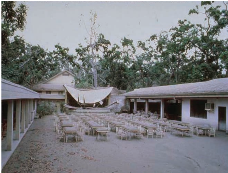
Collapse of a weak metal sheet roof under 150 - 300 mm of ash during the 1991 Pinatubo eruption, Philippines ©T.J. Casadevall, USGS.
