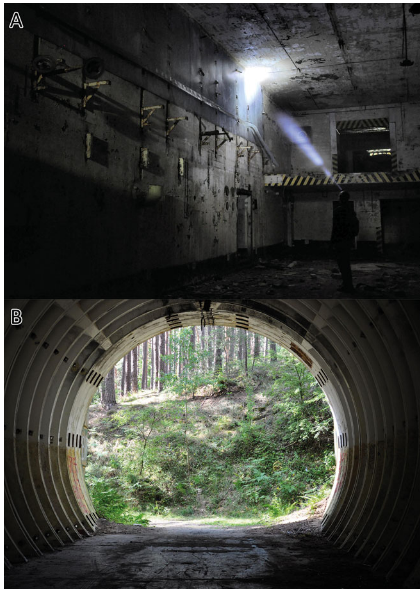
Figure 5. Inside the ruins of abandoned nuclear bases (present day). (A) The main hall of the T-7 warehouse at Object 3003 in Templewo; (B) Ruined Granit warehouse at Object 3002 in Brzeźnica-Kolonia.
